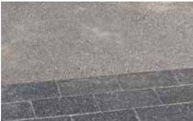
Use non-flexible restraint such as concrete, steel edging or pavers. Ensure top profile of compacted Pathway Aggregate is higher than top of edge restraint to allow watershed.
